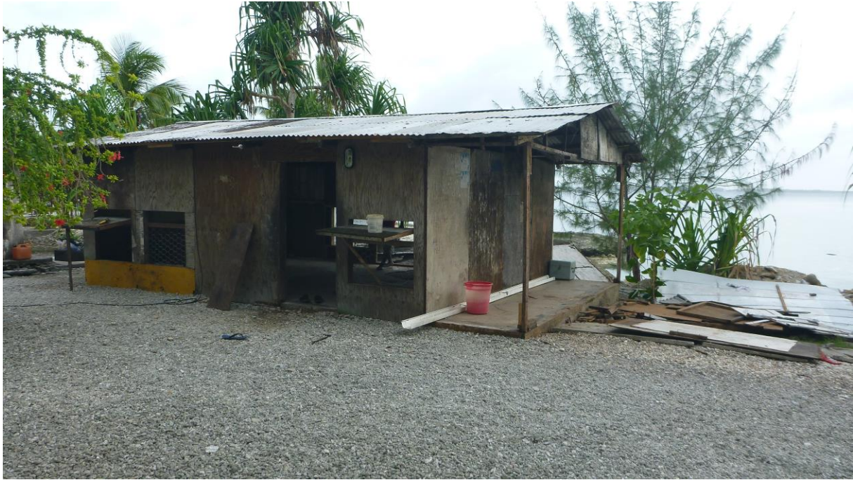
Photo 5. Diminished American-style house. This Rearlaplap house has diminished by the length of the exposed concrete foundation (right-hand side), following the removal of waterlogged parts.
