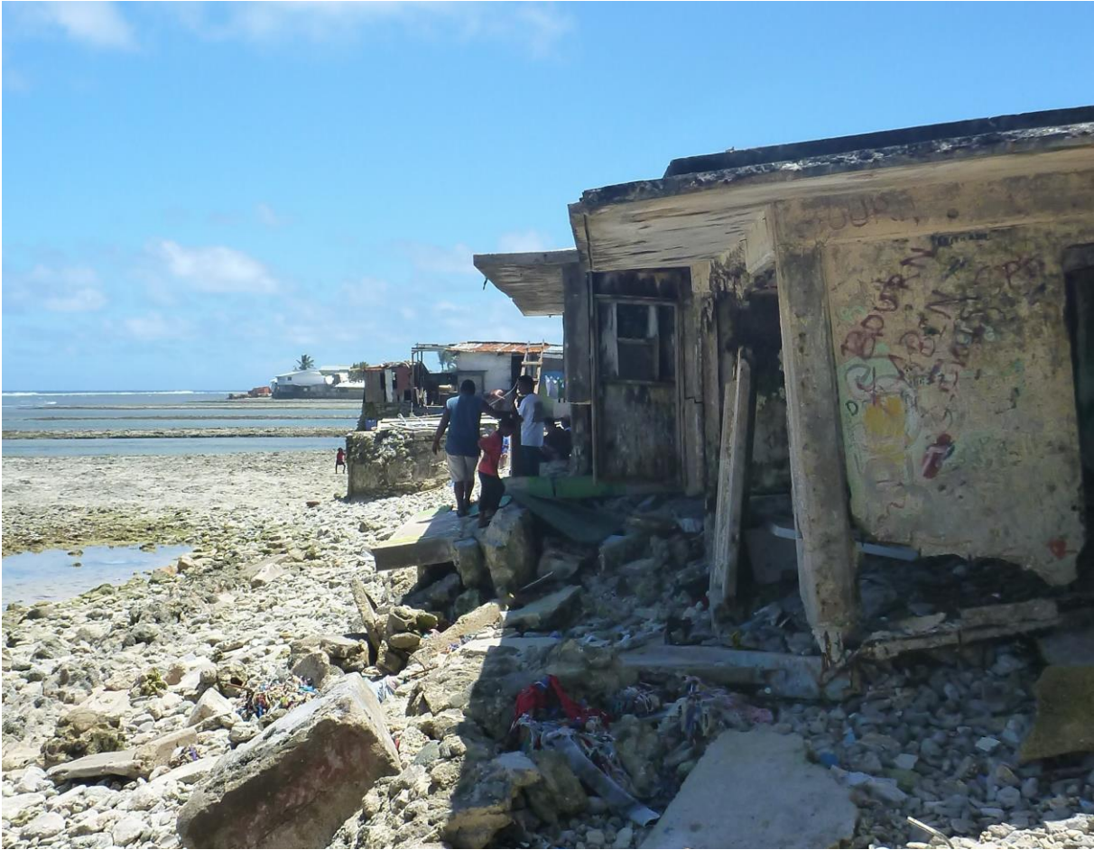
Photo 2. Eroded foundations. The structural integrity of this house on the ocean-side of a Majuro settlement has been weakened, so that the structure has partially collapsed under its own weight.
