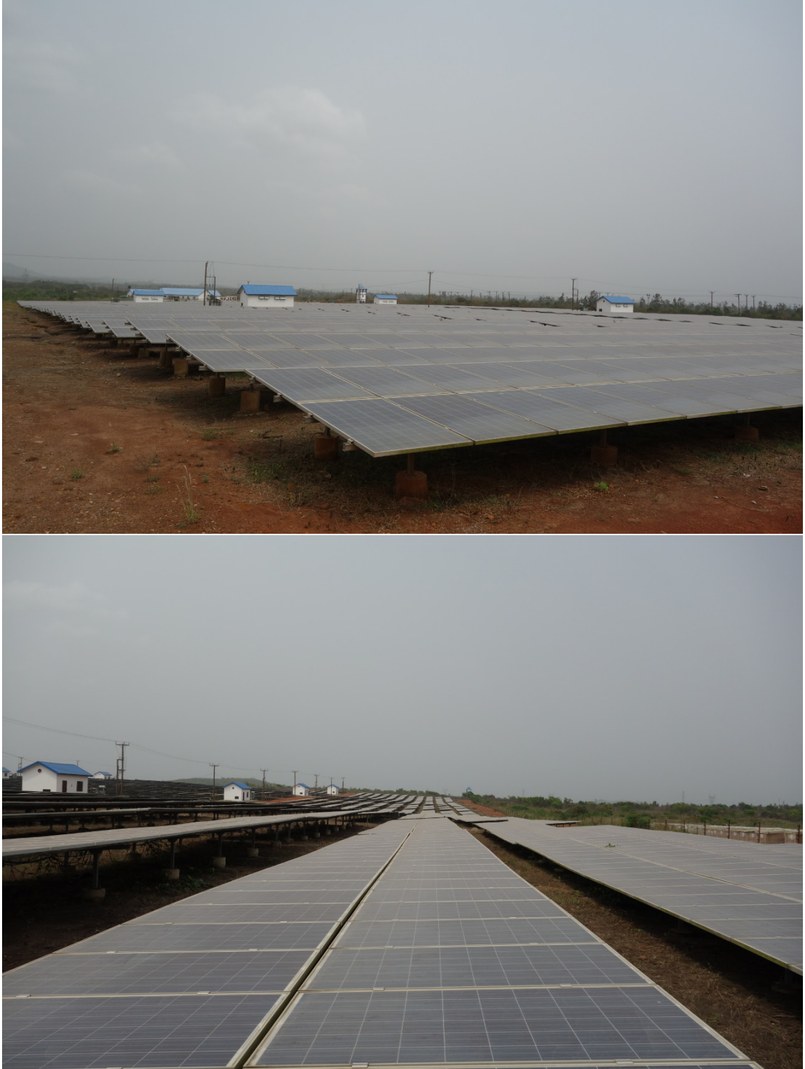
Figure 1.1: Pictures of a solar farm in Ghana. Photo: Daniel Engelsen
