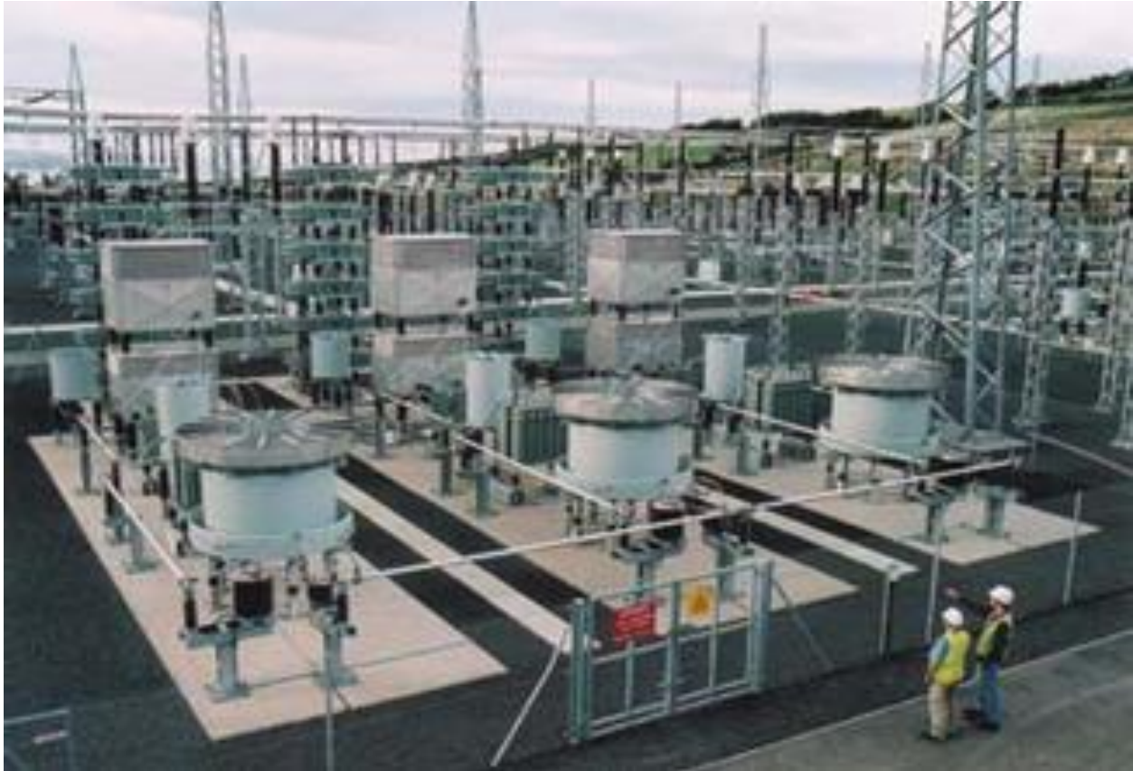
Figure 8.2 AC filters at Moyle HVDC station (2001). From Siemens.
