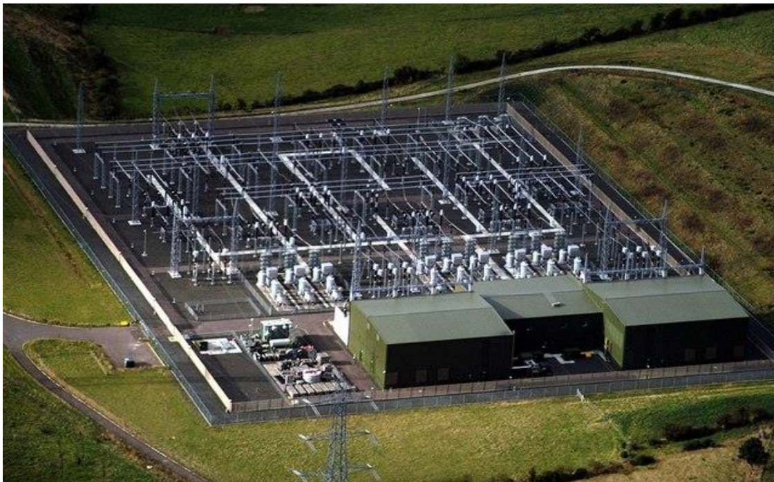
Figure 1.2 Terminal station of Moyle HVDC interconnector (Bipole 2x250MW, \pm 250\text{kV} , with light triggered thyristors, commissioned in 2001). Reproduced with permission of Siemens.
