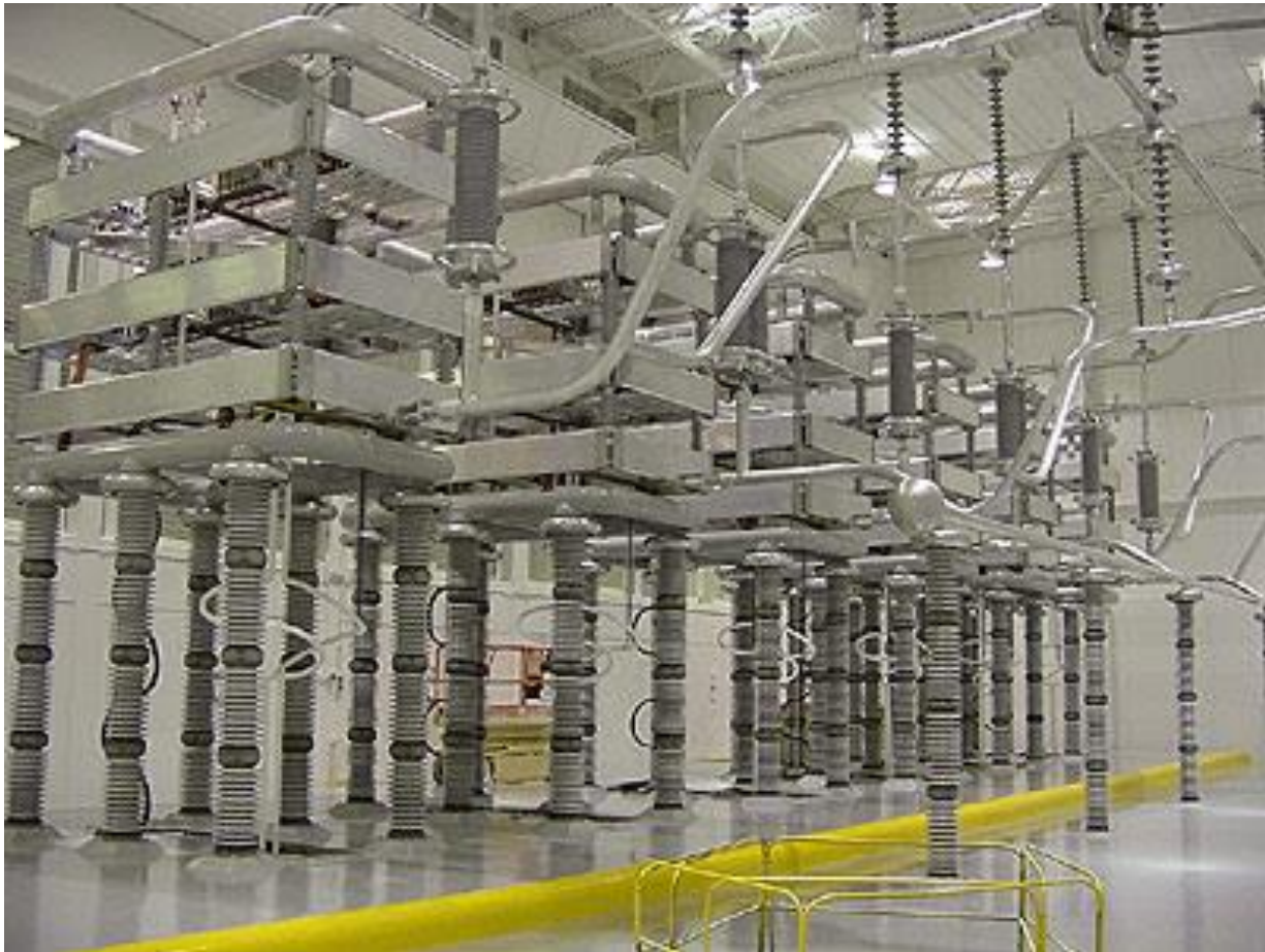
Figure 2.12 HVDC Thyristor valves hall of the Celillio converter Station in the Dalles, Oregon
