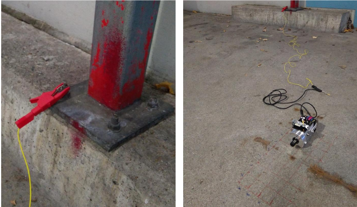
Figure 65: Field test in a parking house with corroded rebars on the concrete floor. The picture to the left shows the ground connection and the picture to the right shows the FKP and the measured area.
