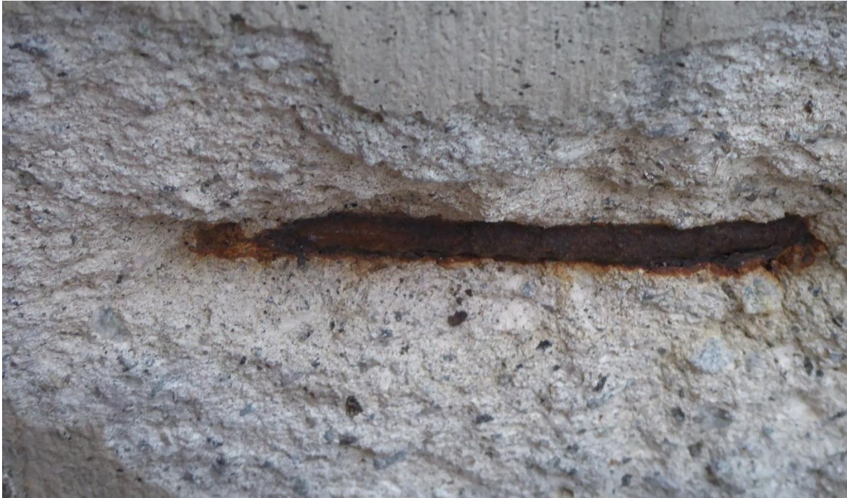
Figure 3: Corrosion-induced cracking has exposed a rebar and resulted in spalling of the concrete wall.
