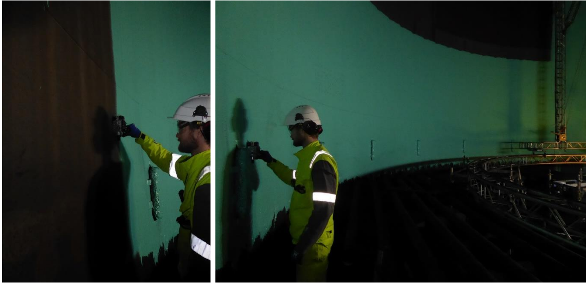
Figure 67: The FKP being used for measurements on the painted (and unpainted) metal surface on the inside of a large storage tank at an oil terminal.
