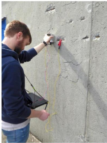
Fig. 7 – A possible way to deploy the FKP on real concrete structures. Here we show an attempt to measure a concrete wall with visible cracks along the rebars. The red-blue wire is used to power the instrument (battery pack in the operator's pocket). The yellow wire connects the FKP to the ground (i.e. one of the rebars).
