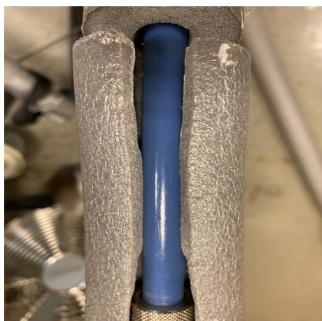
(a) Before cleaning.
