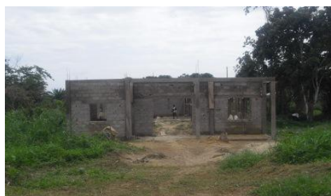
Photo 5.4 uncompleted community hall at Lobe
