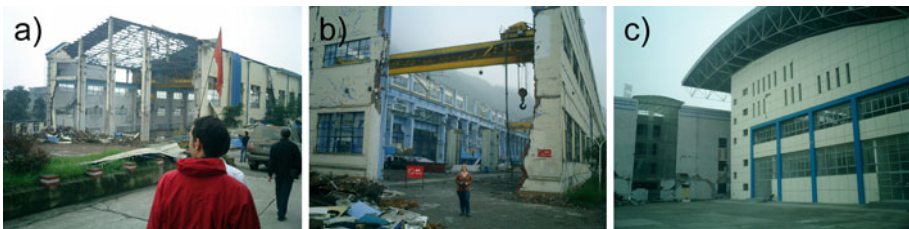
Fig. 12 Factory buildings of the Dong Fang Steam Turbine Factory. a–b Older factory buildings, which suffered from substantial damage as roof collapse. c The gymnasium of the factory, which is a newer steel structure, had no apparent damage after the earthquake
