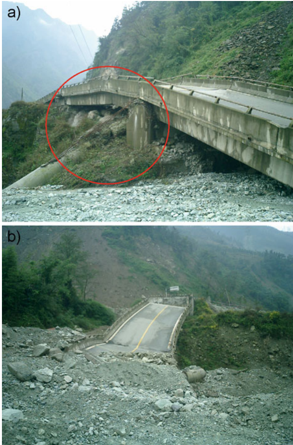
Fig. 11 Structural damage to the highway between Chengdu and Yingxiu. a View towards Chengdu. A collapsed column is visible in the lower left corner. b View towards Yingxiu, where the road section in the foreground is dislocated and separated from the section in the background
