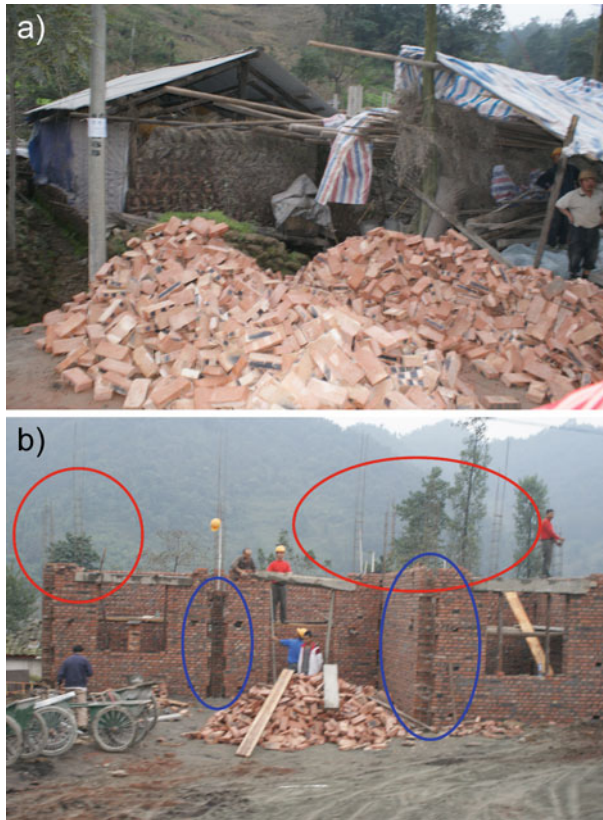
Fig. 23 Reconstruction work near Bailu. a Piles of bricks visible along the road. b Construction of simple reinforced concrete building with brick infill. Notice the concrete columns in the corners ( marked with blue and red circles ) are until now only visible due to the simple metal structure, while the concrete columns have not yet been made
