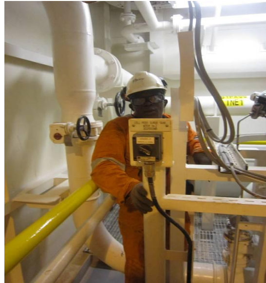
Plate 14: Appropriate men's work: a pumpman doing repair work in the pump room on a rig
