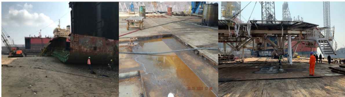
Priya Blue Industries Private Limited [1]: landing area/ drainage facilities/ secondary cutting deck.
