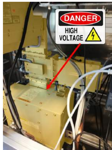
Figure 15: Do not touch the regions shown in yellow, nor any connected metal surfaces that aren't grounded.
