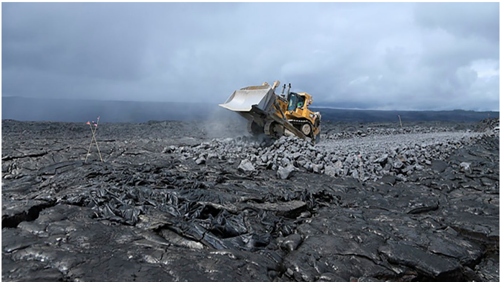
FIGURE 5.3: Road workers are bulldozing a road through the lava fields between Kalapana and the Chain of Craters Road in Volcanoes National Park in 2014. Photo by NPS Photo/David Boyle.
