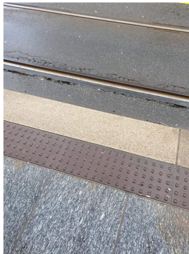
Figure 5.6: This tile often gets slippery when it is wet
