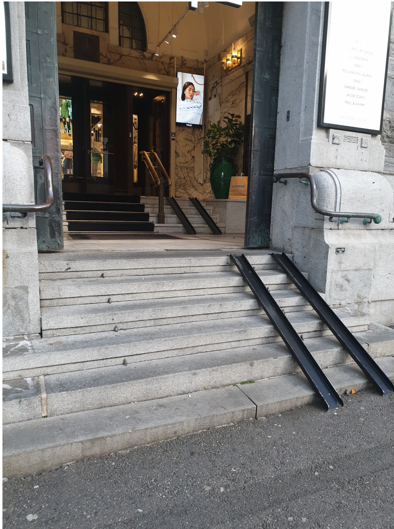
Figure 6.2: Too steep ramp which is in the way of the bad hand rail
