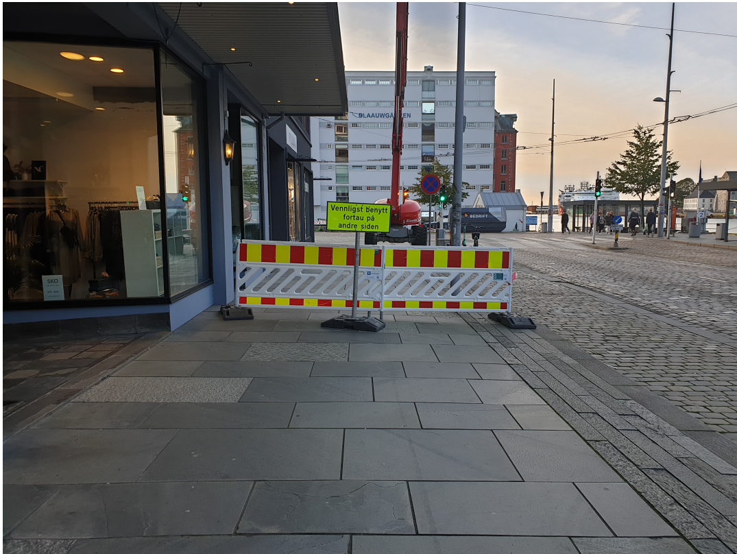
Figure 6.6: The sidewalk is blocked by construction
