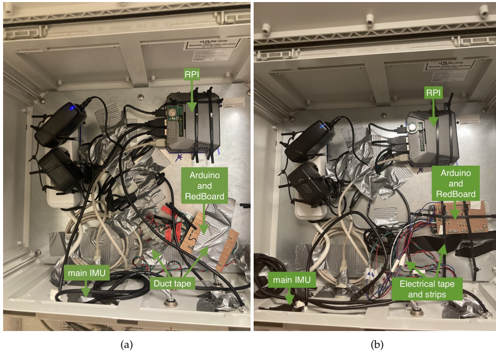
Figure 6: Picture of (a) the original processing unit operating until 29.04.22 and (b) the new processing unit operating from 15.09.22. The system components are identical, but the new unit is mounted with strips and electrical tape instead of duct tape.
