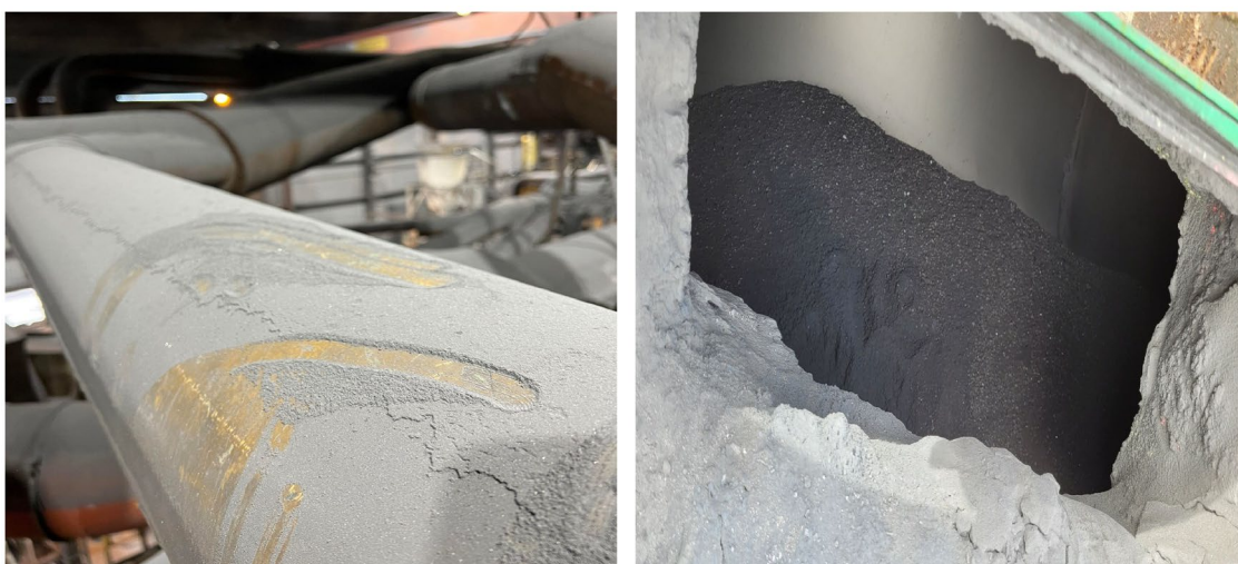
Figure 2: Dust layer on top of dust extraction duct (left). Dust deposits inside dust extraction duct (right). Bjølvfossen 9. June 2022.
