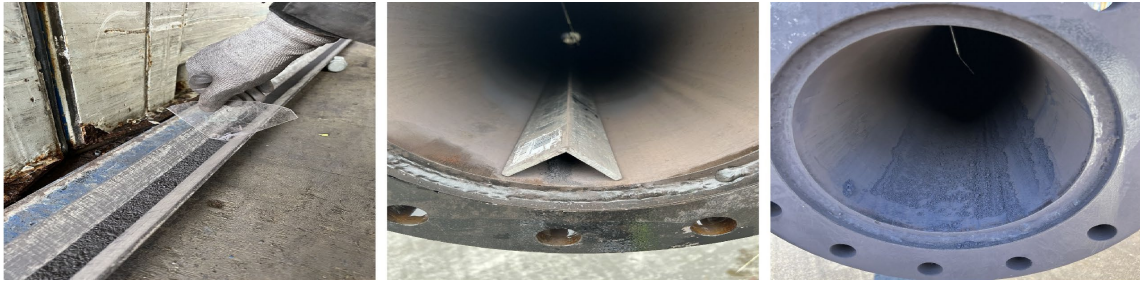
Figure 24: Illustrating the distribution of dust in the angle iron and in the DN250 pipe.
