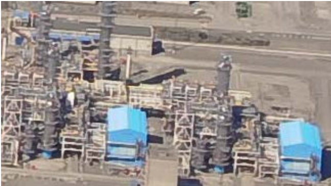
Figure 17 Åsgard processing trains
