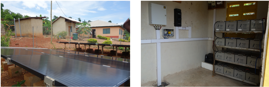
(a) A microgrid installation in Kofihwikrom, with the local medical clinic in the background. (b) The power converter room with batteries for electrical storage.
