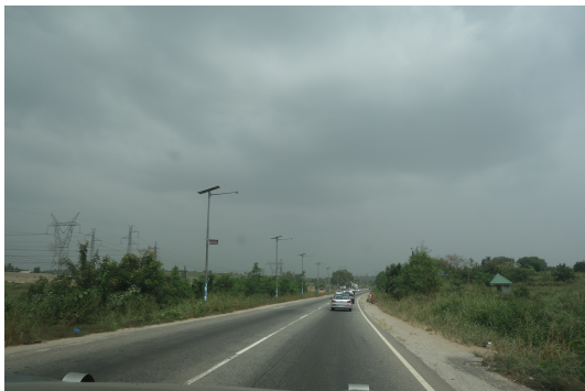
(a) LED street lights powered by solar panels along a main road in Ghana.
