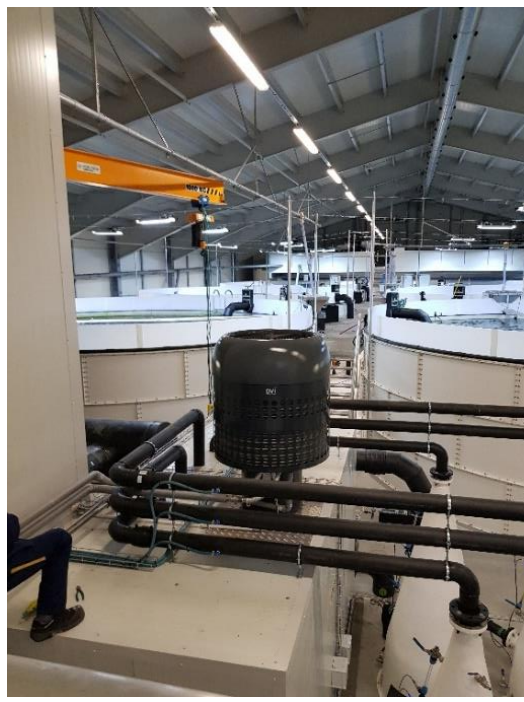
Figure 5 - Tanks in room 2
