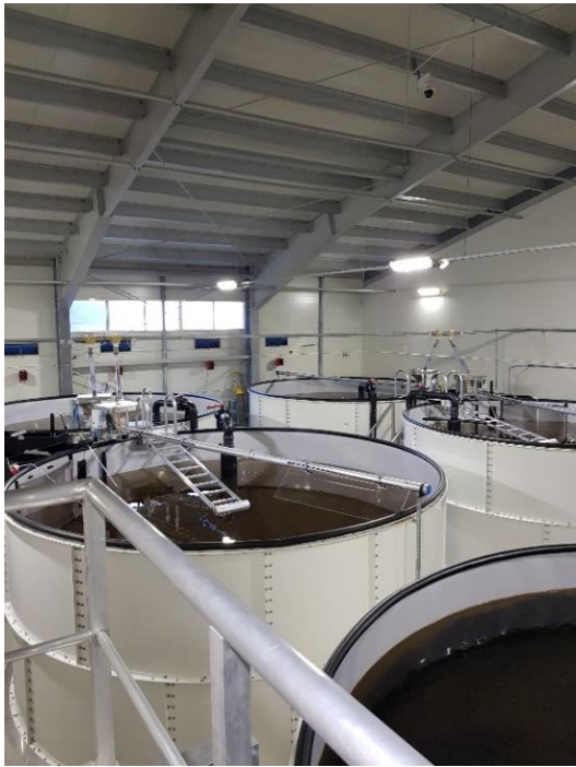
Figure 4 - Tanks in room 1
