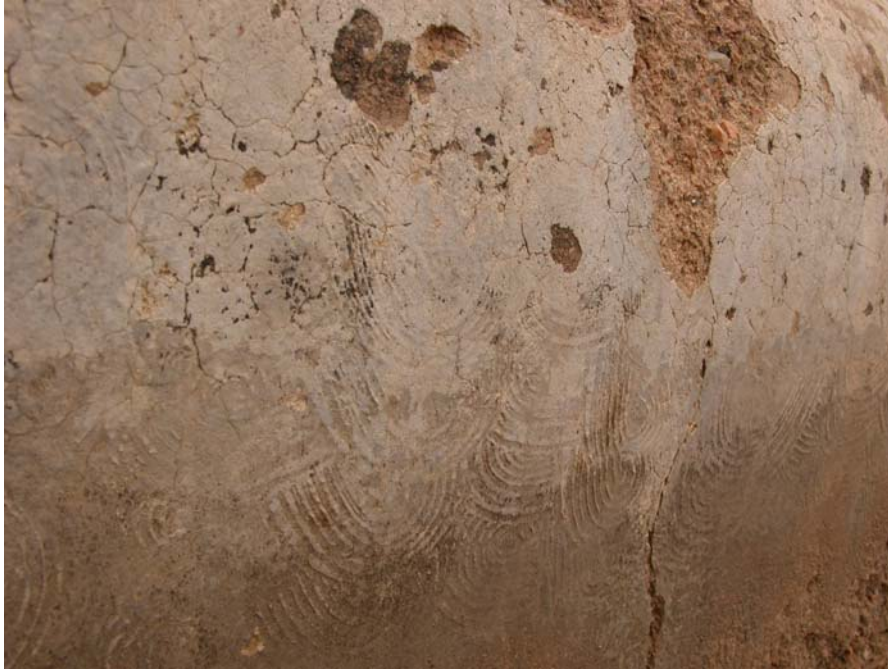
Fig. 28 Birkat al-Ḍahrayn, city of Hajja. The final layer of nura has been given 8-shaped brush strokes. This proves it was not polished. Some very simple cisterns do however have polished parts. This is taken just above the water line and in the lower right corner one can see the etching of the water. A similar pattern was found on other cisterns.
