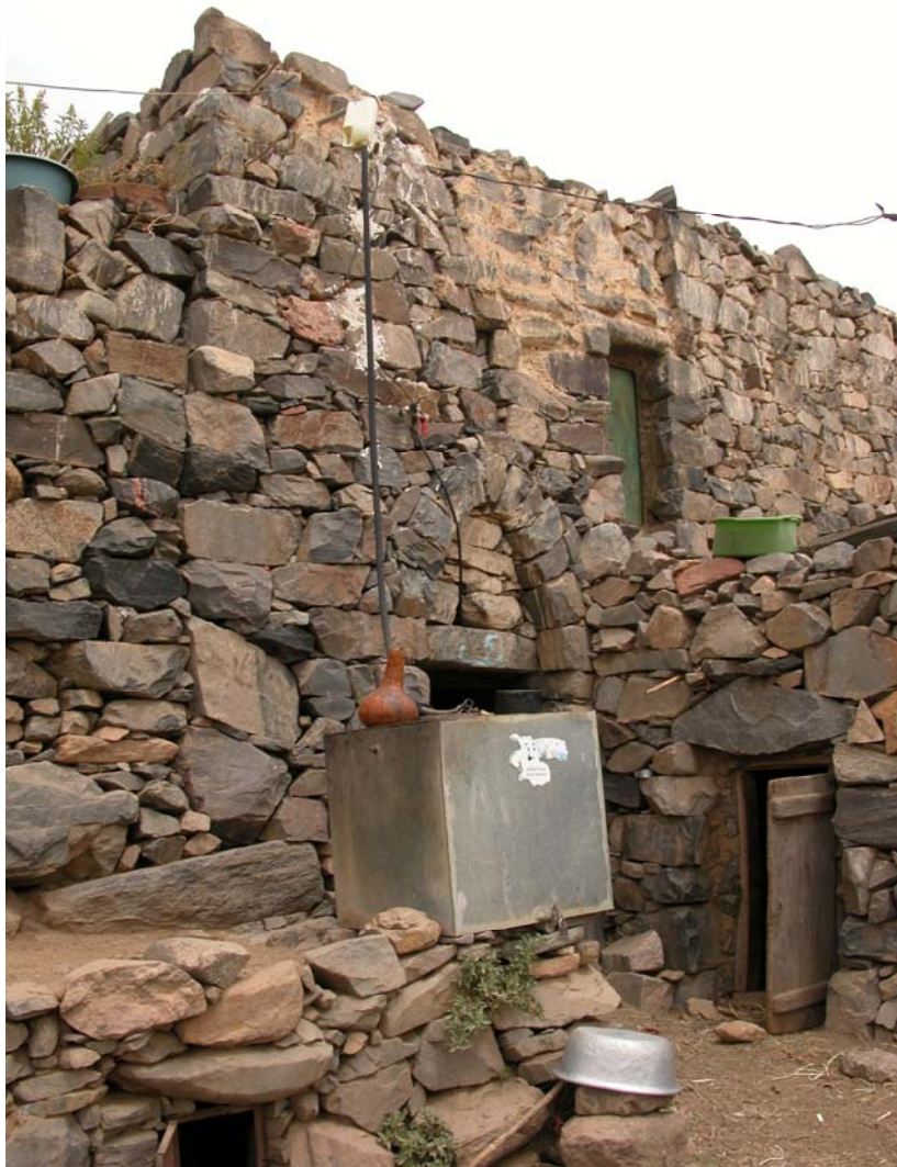
Fig. 9. Roof water harvesting is found in the field area, but is not very common. Problems of private nearby storage capacity and small roofs compared to the house size, are problems mentioned by the informants. The drainage pattern on old houses is also a problem; the walls in the houses project up through the roofs and divide the roofs into sections that each drain through different gutters on each side of the houses. Old roofs also have sand cover that will not produce as much and as clean runoff as concrete. There is a small tap on the water tank and it is always locked with a small padlock. Note the pots with herbs and flowers on the side-roof; the roof is namely the only flat, goat-free surface and may be used for many different activities, including drying clothes and out-of-reach storage. According to informants, this is one of the reasons for the general lack of roof water harvesting.
