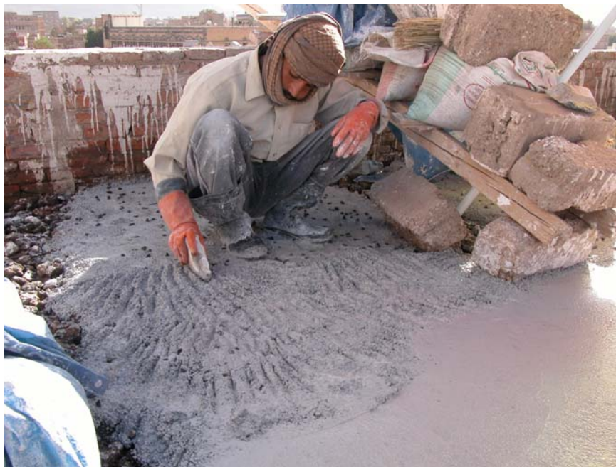
Fig. 27 Beating the first layer of qadad into the surface of gravel under. The picture is taken of a construction of a new roof in a traditional way in Sana'a. The beating is done systematically with a semi sharp edge. The part in the right corner has been beaten enough and has been made smooth. The layer is circa 5 cm thick.
