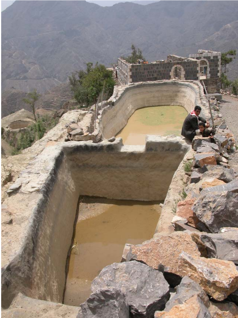
Fig. 24 Private cistern with a very large settlement basin. The runoff comes from a road.
