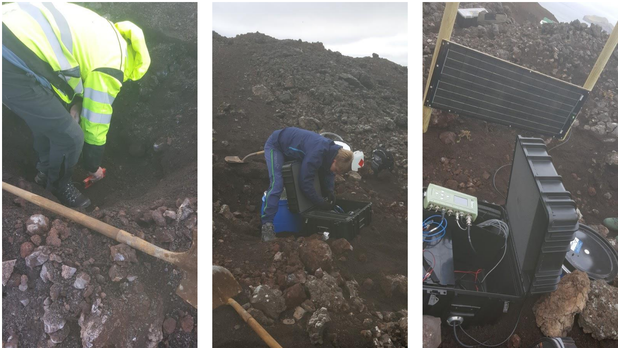
Figure 9.1: Additional pictures from the field installations of HEM1.
