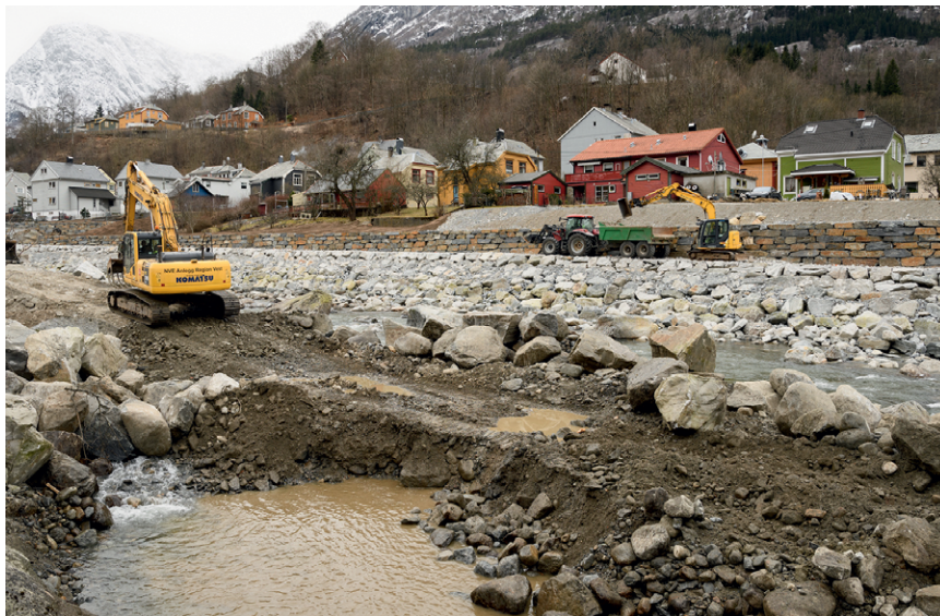
FIG. 3. During a visit to Odda in Mar 2017, some of the Hordaklim researchers got to see the extensive repairs being done to the River Opo after the flooding episode in Oct 2014 (Pontoppidan et al. 2017). Photo by Erik Kolstad.
