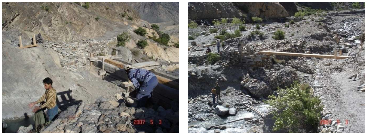
Photo 5. 1 Public participation to construct bridge on local river (Ghang Kyu) of Thini
