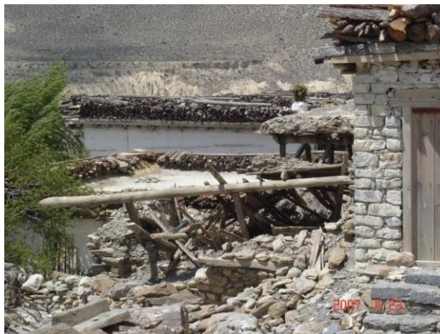
Photo 8. 2 A damaged house: Waiting for Poorji
