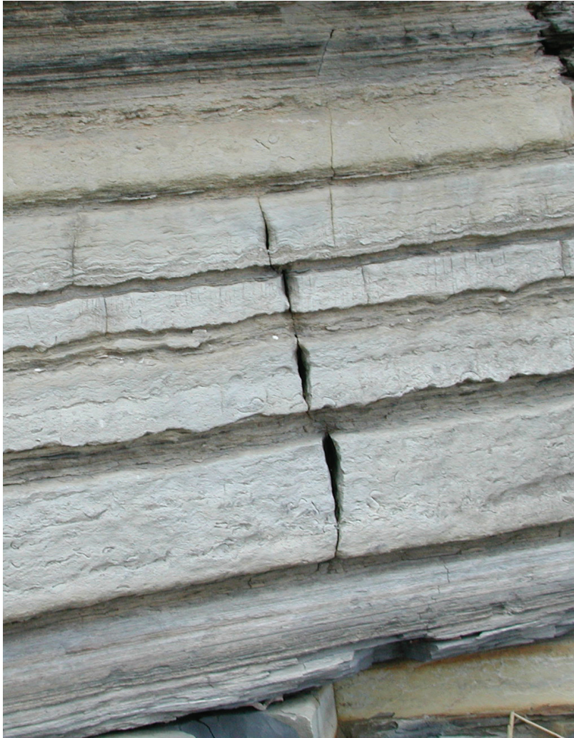
Figure 3.5: An original extension fracture cutting through a succession of limestone and shale has resulted in vuggy fractures after being subject to dissolution at Lavernock Point, South Wales. The limestone layers are the ones most affected by dissolution. The length or dip dimension of the extension fracture is approximately 50 cm.
