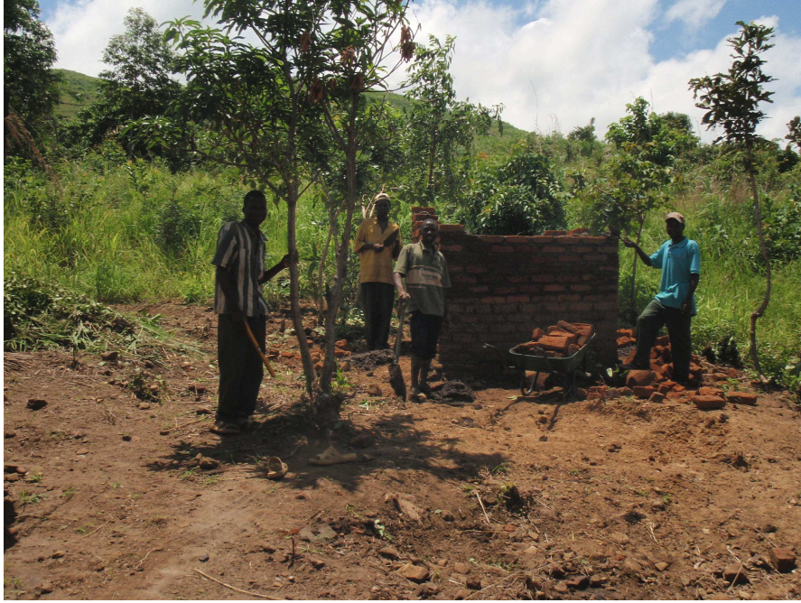
Photo 4: Members of a VHC building a pit-latrine for an outreach maternity ward.
