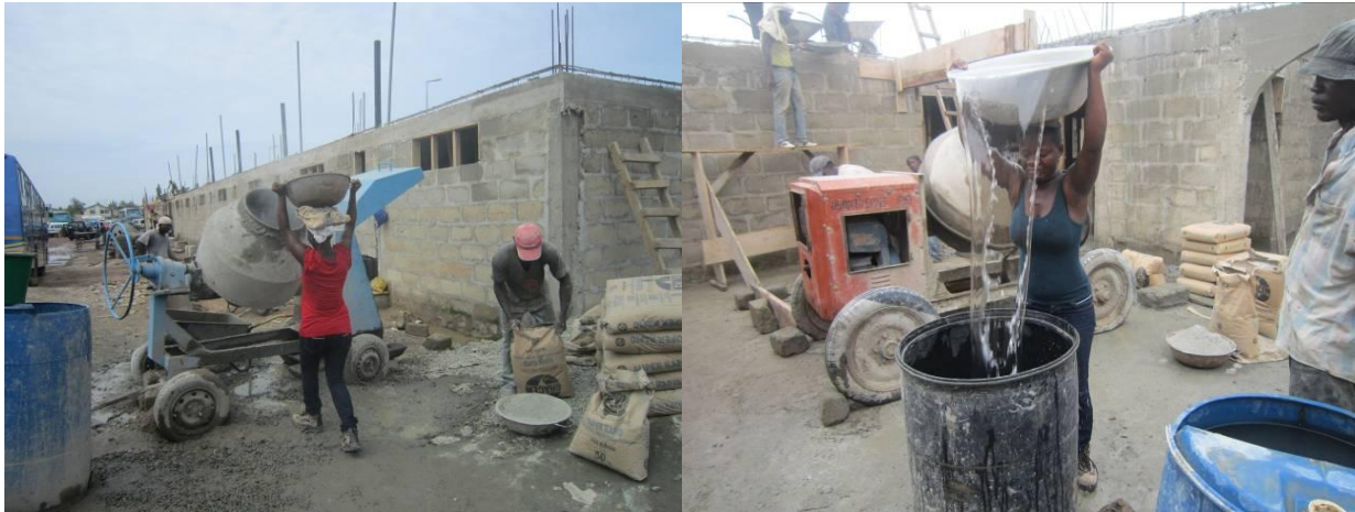
Plate 3: Carrying sand into a concrete mixer machine. Plate 4: Pouring water into a water container.
