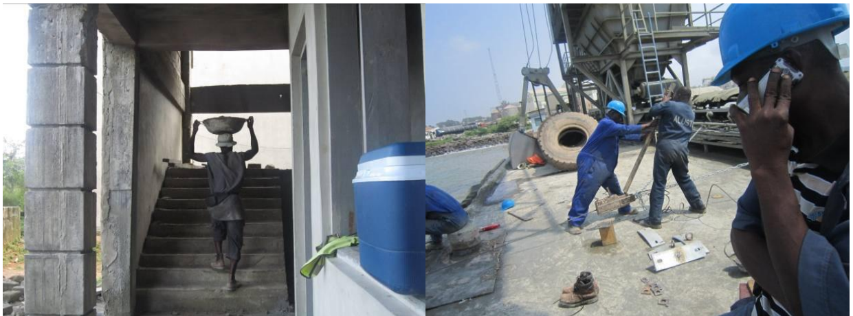
Plate 20: Carrying concrete to the next floor. Plate 21: Wharf making at the port, foreman on phone.
