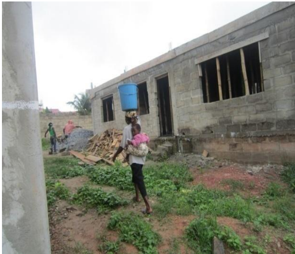
Plate 14: Woman with baby at the back carrying water at a construction site.
