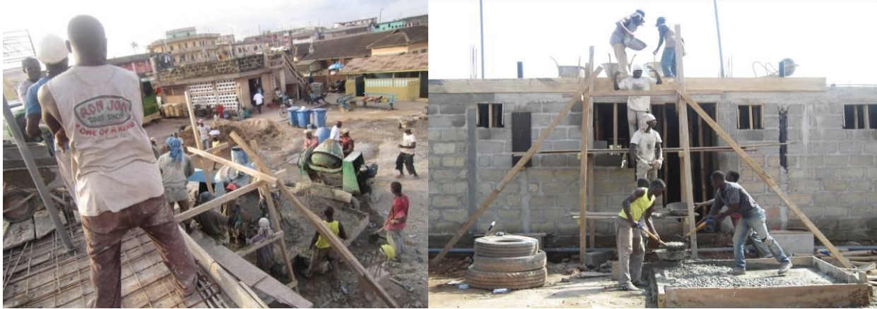
Plate 18: Working, concrete mixing machine in the background. Plate 19: Carrying concrete to the next floor.
