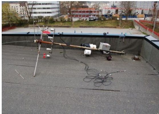
Figure 5.4: Vandalism of the AWS at Haukeland Elementary School during Easter 2011.
