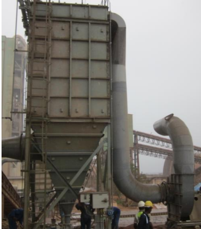
Figure 3: Bag filter dust suppression system in the old crusher (Photo by Tungu)
