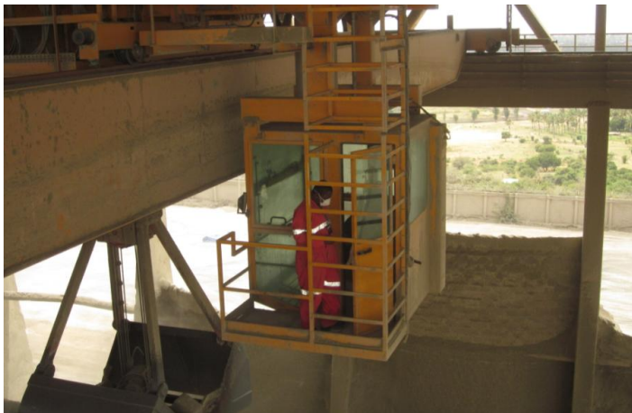
Figure 5: A crane operator entering the overhead crane cabin in the old production line (Photo by Tungu)
