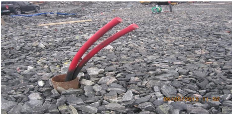
Figure 2.5: Top end of down hole heat exchanger in Åsane
