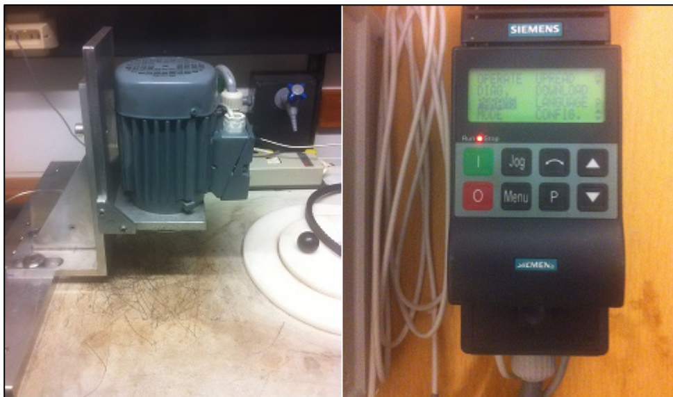
Figure 3.4: The VEM GmbH electric motor to the left is controlled by the Siemens MICROMASTER inverter to the right.
