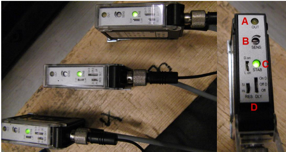
Figure A-6: Flame detector amplifiers. A: signal out indication (detection), B: Sensitivity, C: Stability (here: yes), D: Resolution and Delay settings.
