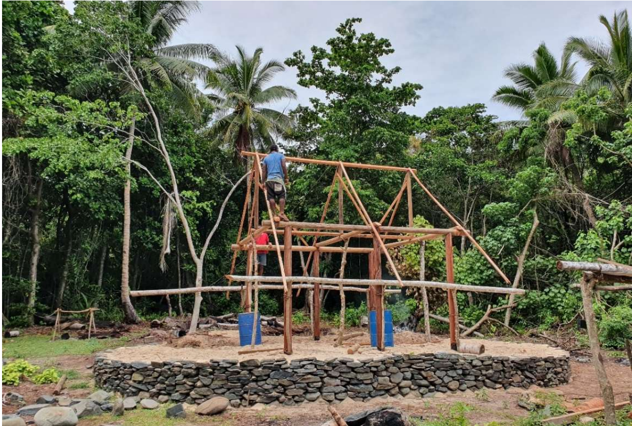
Figure 5 Early stages of construction as carpenters were making the framework of the bure at Selavo. Photo by author.
