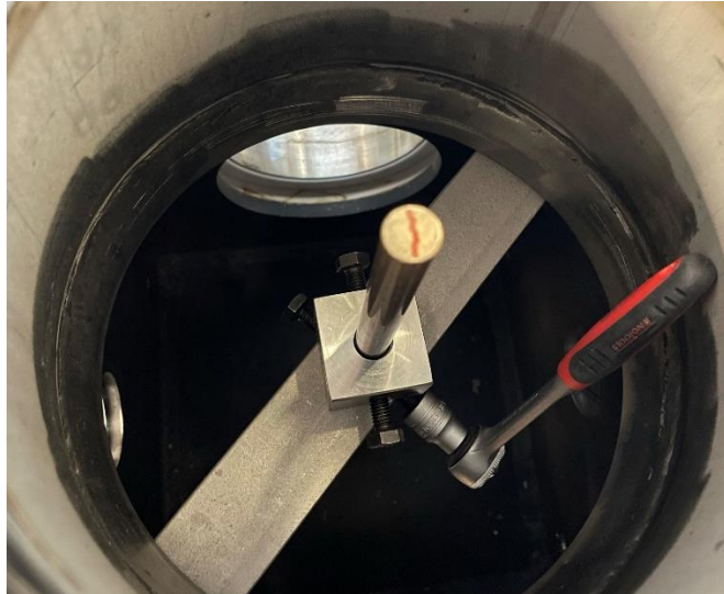
Figure 4-10: The connection rod installed in the transverse steel beam – the socket wrench operates the set screw fixing the connection rod to the beam.
