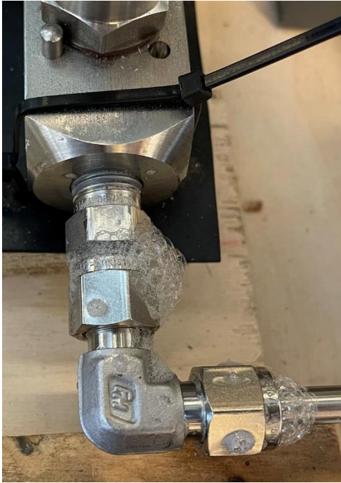
Figure 4-8: An example of two minor leakages identified with bubbling soap film at approximately 100 bar nitrogen pressure.
