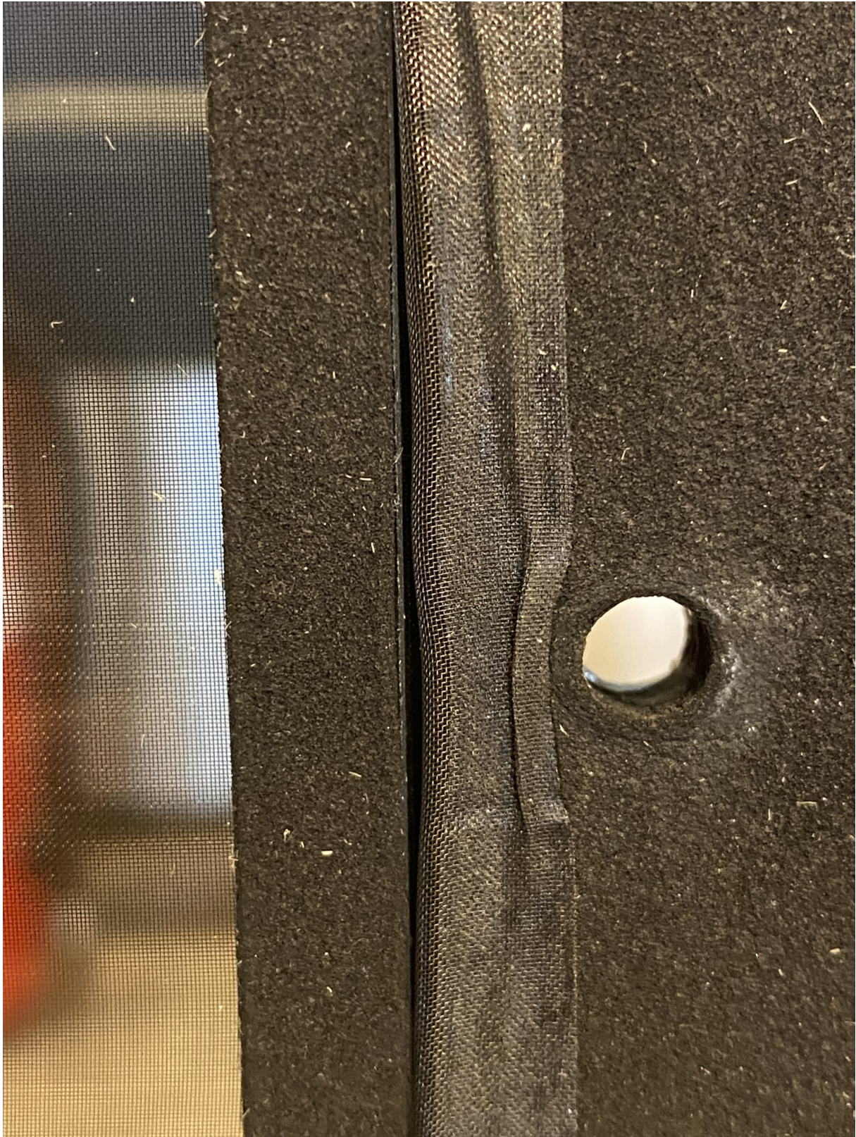
Figure C.4: Improved windows, close-up view of rubber/foam gaskets connecting laminated mesh to faraday cage. Photo: Daniel Asle Vingen Endal.
