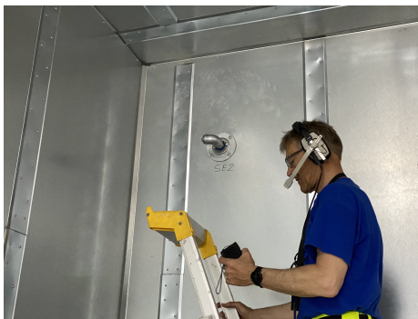
(a) SE for NOVEC fire suppression system.
