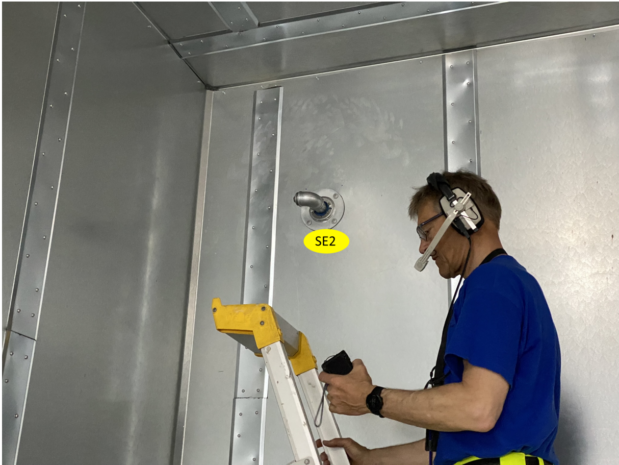
Figure C.3: Single entry for the NOVAC fire suppression system. Photo: Daniel Asle Vingen Endal.
