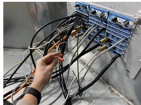
(b) SE for cable pass-through. Viewed from inside Faraday cage.
