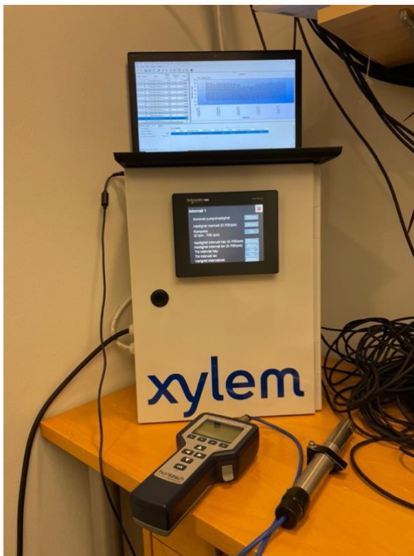
Figure 17. The set-up of the PLC with the handheld flow meter and associated flow sensor underneath.
