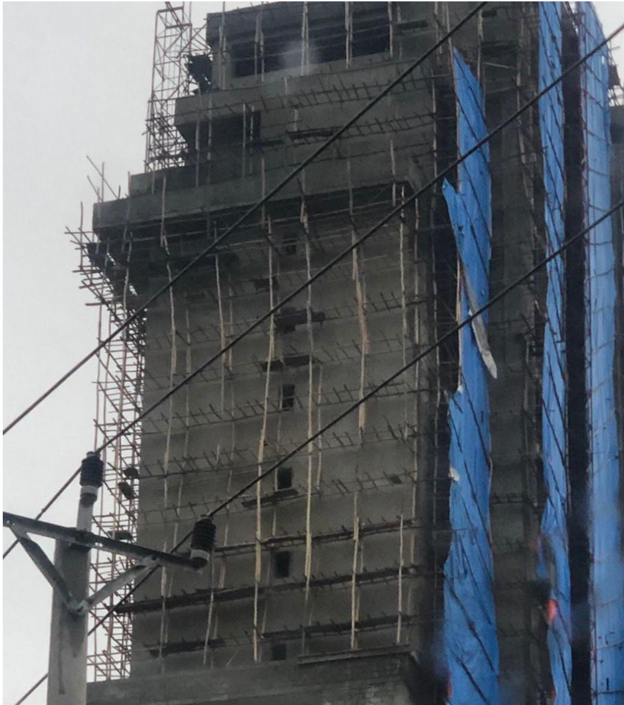
Figure 2. A skyscraper building under construction in Addis Ababa, Ethiopia showing the use of weak scaffolds made of wood. Photo: Tsegazeab Laeke.
