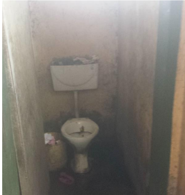
Image 15: A dirty water closet stained with urine and faecal matter at a peri-urban market. This was the state of facilities at most of the markets visited.
