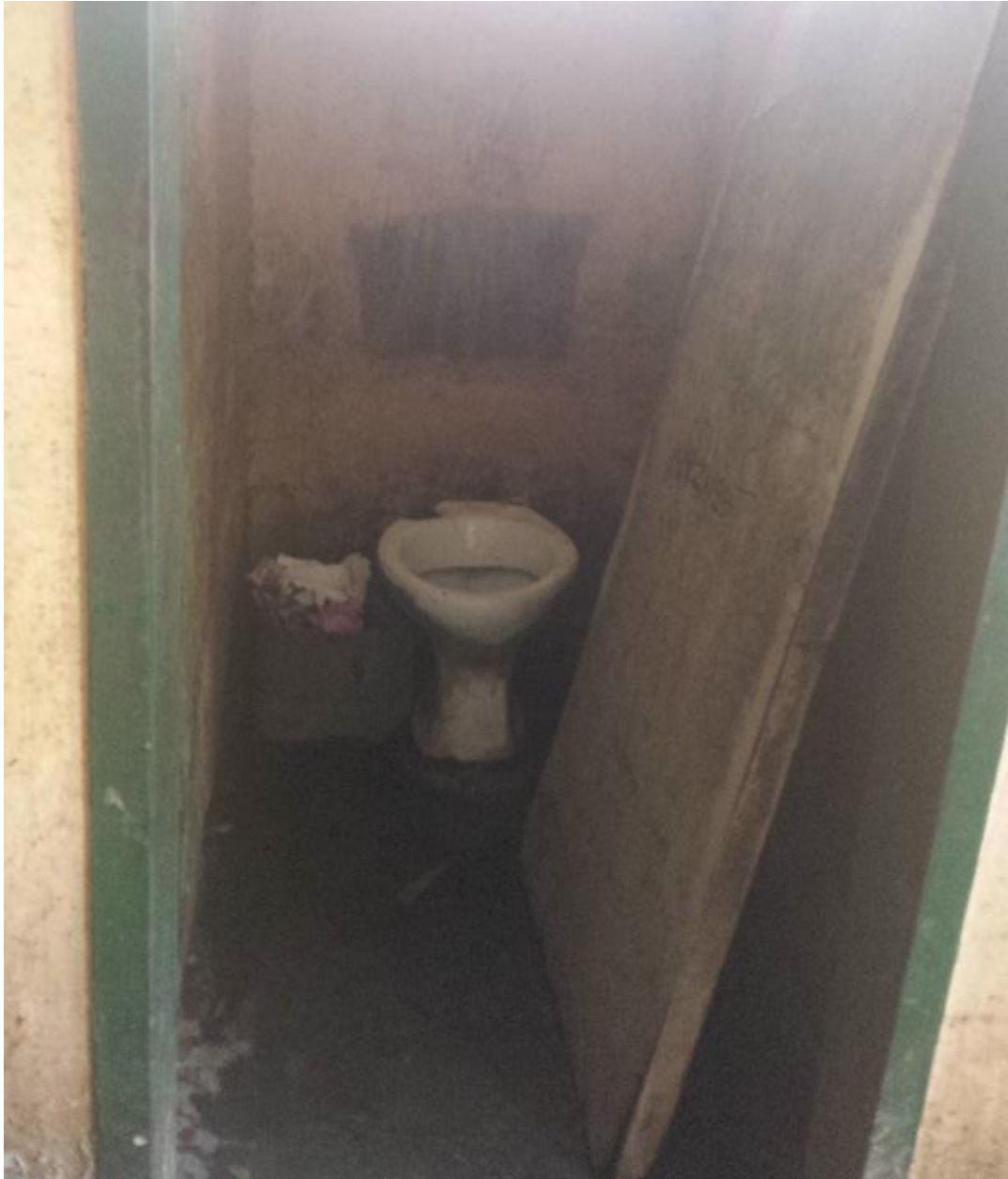
Image 17: Lack of privacy at one of the peri-urban market visited a toilet cubicle with broken door. Traders had to hold the door whilst using the toilet this was the condition of the doors in most of the markets visited.
