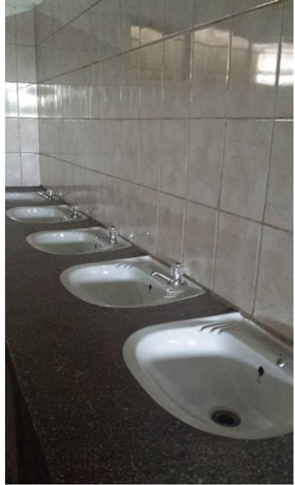
Image 8: Wash hand basins
