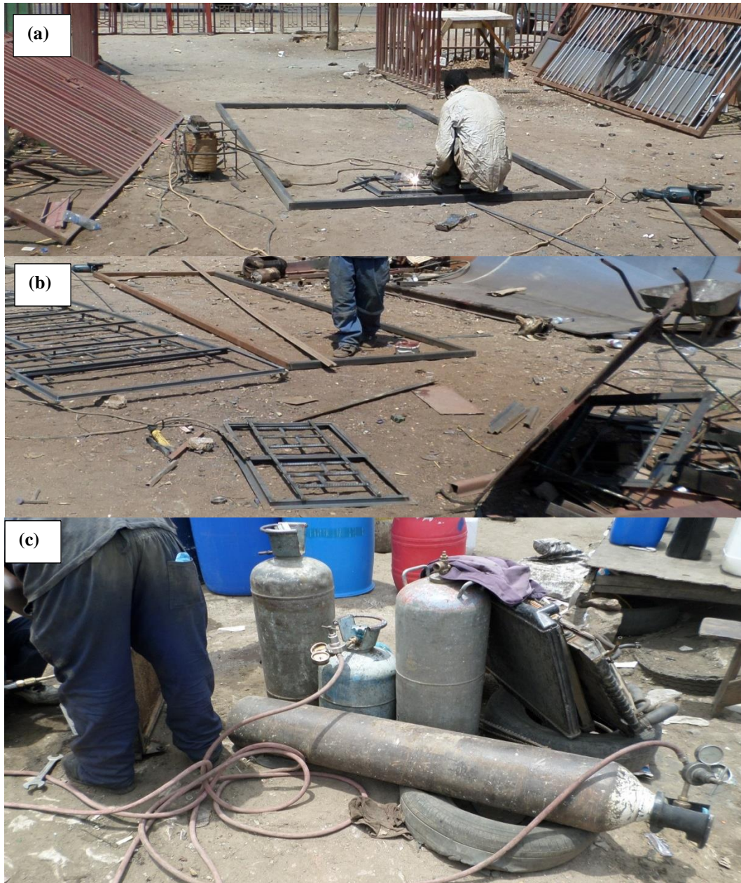
Figure 8: Work Environment Hazards Observed
