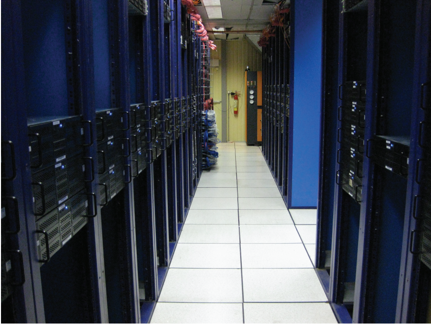
Figure 4.5.: Picture of counting room 2 at the ALICE experiment where the HLT is located. In the racks, FEP machines are the ones in the middle and compute nodes are in the top where also the fibers from the experiment can be seen. Switches and infrastructure nodes are placed in 4 racks to the left at the very far end of the two rows seen in the picture.
