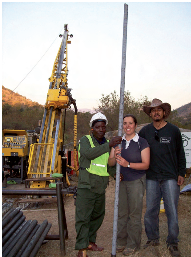
Figure 2. Drill rig aligned and set to drill at the shallowest possible angle ( 45^{\circ} ) relative to the dip and dip direction of the steep near-vertical orientation of the geological units along the Komati River. The >3-m-long rod is composed of basalt or diamictites.
