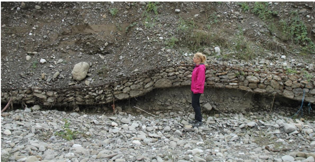
Figure 3.2: An example of how the man made netting cages forming the artificial embankments looks like. Here from the lower parts of the Inahos fan.
