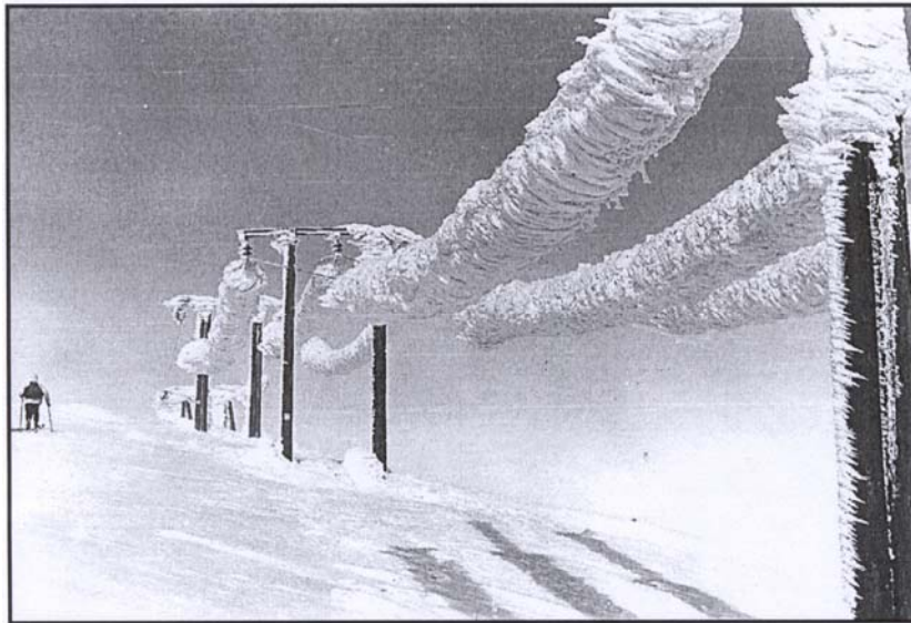
Figure 1.1. Rime on a 22 kV overhead line at Voss, Norway on April 18, 1961. Ice-load recorded was 305 \text{ kg m}^{-1} on each span. (photo: Olav Wist).
