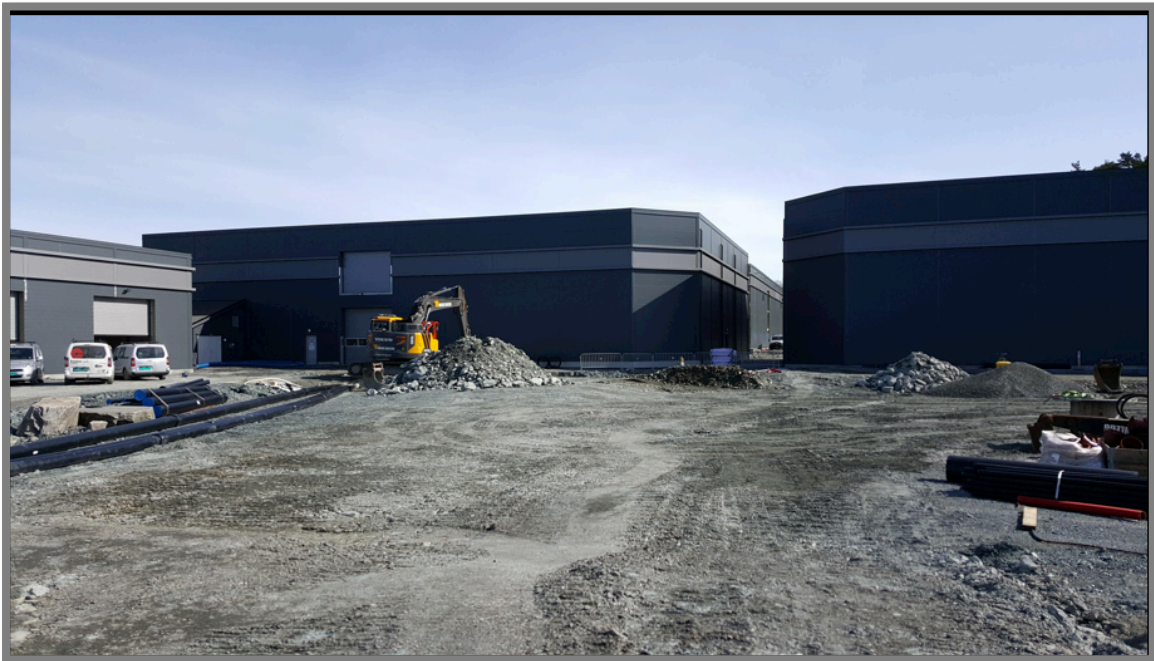
Figure 1: Two RAS modules at Erko Settefisk AS. The technology and module concept were delivery by Nofitech AS. Photo: Karine Drønen
