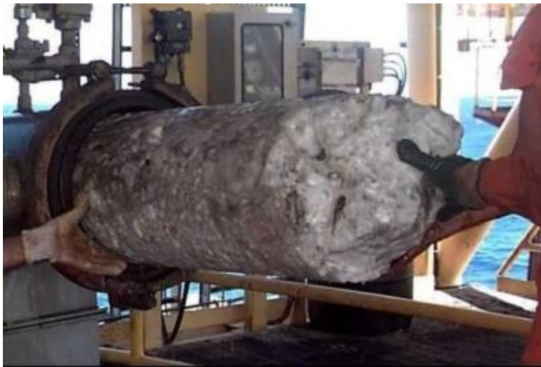
Figure 1-1: Pipeline plugged by gas hydrates (4) .
