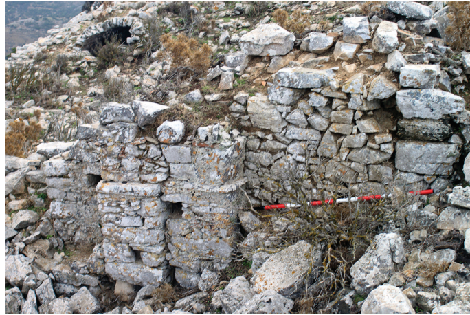
Figure 4. Piers inserted on the southern wall of Building A, probably connected to rebuilding the roof.
