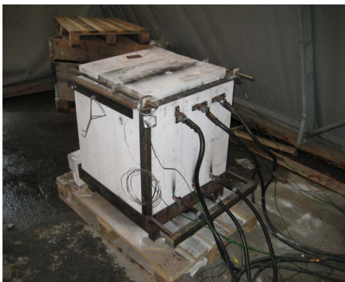
Picture 4 shows the furnace from behind where the power cables are connected to the copper plates
