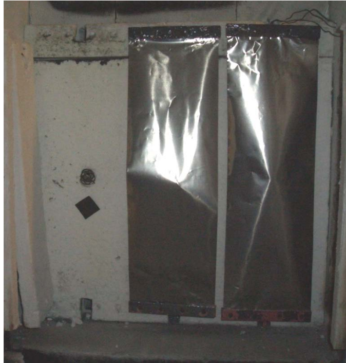
Picture 7 shows one of the installed foil bits placed against the isolation as a small square on the left side. The thermocouple, designed as a spring, measuring the surface temperature on the radiation foil can be seen above the foil bit.
