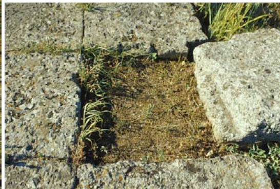
Figure 2.8 Adjustment of one of the Archaic foundation blocks into the foundations for the wall between the opisthodomus and the cella of the Classical temple.
