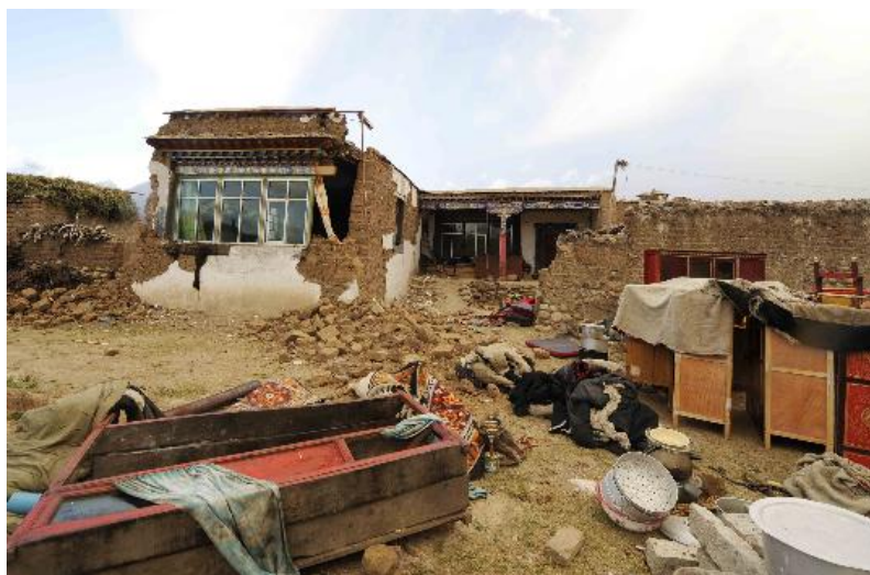
Figure 3.5 A damaged house in Gedar village, Damxung, Tibet, on 6 October, 2008. From Xinhua news agency.
