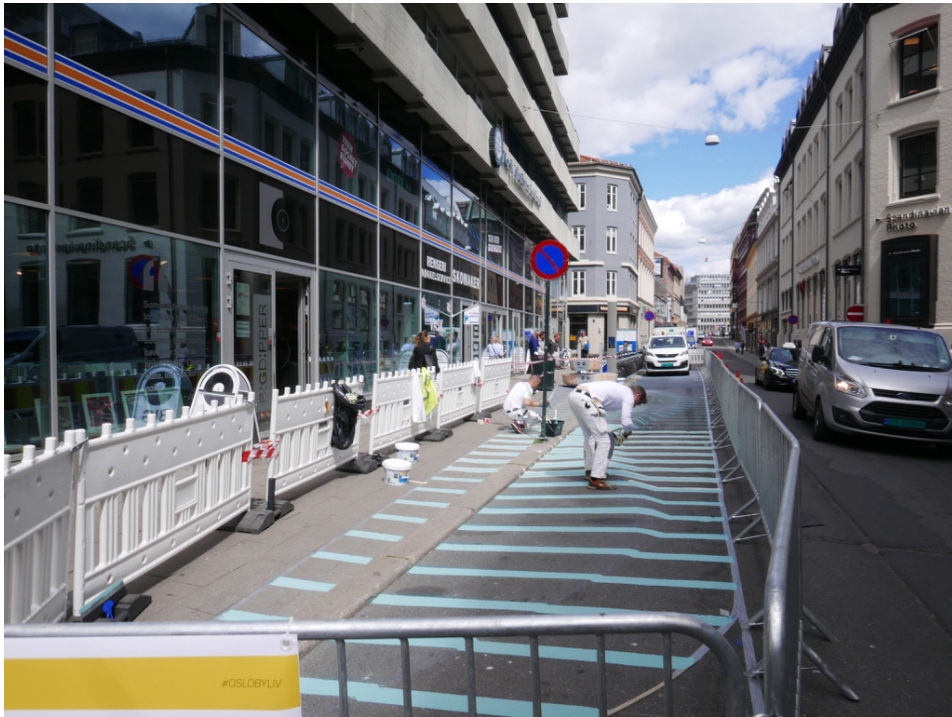
Figure 6: Implementation of temporary measures and use of street furniture to create a car free city centre through the "Bilfritt byliv" project (photograph by the author).
