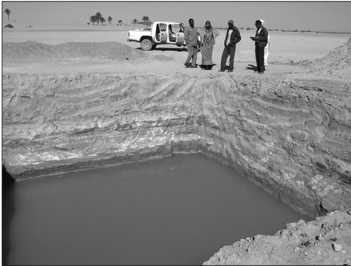
Plate 2.4: A Trench Dug to Erect Wireless Tower at Wadi al ga'ab Shows Water at 3 Meters Deep
