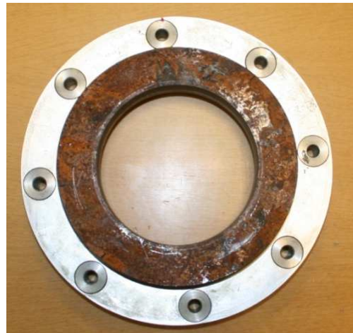
Figure 2-28: Picture of the plane rusted flange mounted on the flange adapter. From (Opsvik 2010)
