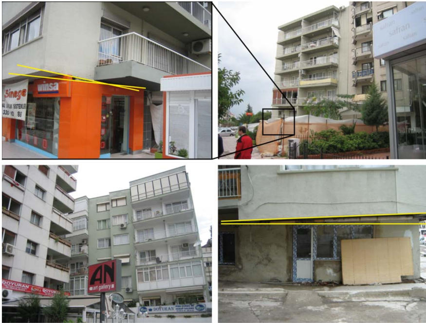
Figure 18. Pictures of houses in the Karşıyaka, district of İzmir. Tilting of the structures due to soft soil conditions is visible. The picture at the lower right is from the rear of the house shown in the upper row. The angle between the yellow lines is approximately 10-15°.
